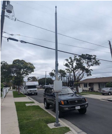
Pole-mounted, solar/mains power, weather-proof.
